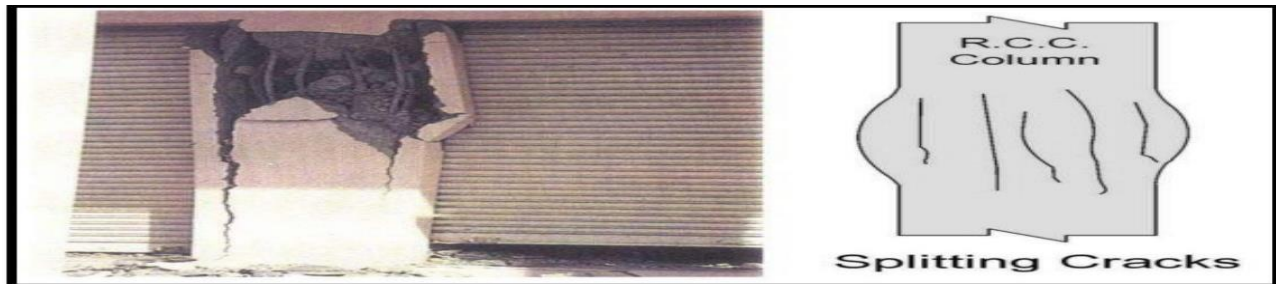
Figure 3: Splitting Crack In The Concrete Column [9] [4]
