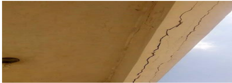
(Cracks parallel to the main reinforcing skewers due to rust)
