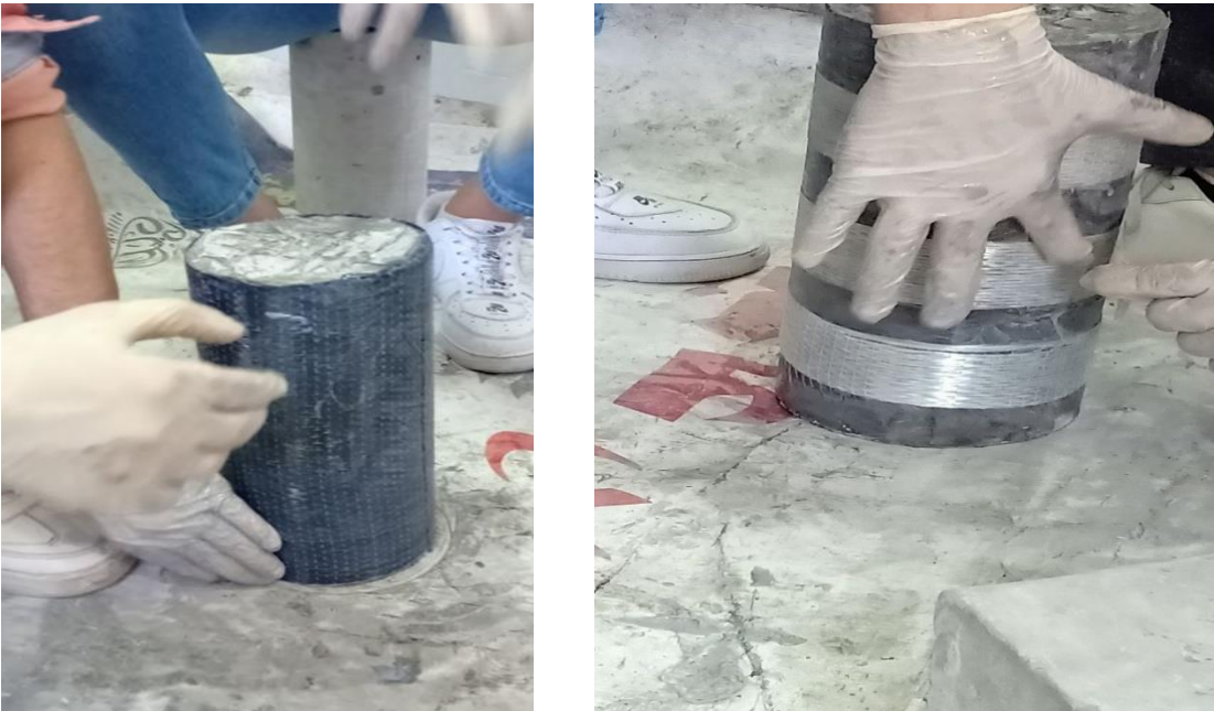
Figure (3-29-d): GFRP sheets and CFRP sheets installing and preparing the surface for the GFRP sheets and CFRP sheets
